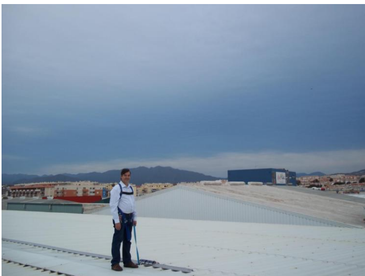
Skyway on top in Malaga – Maintenance Manager Miguel is delighted with the Skyway Safetraxx System on the roof of the Dunnes Stores building.
